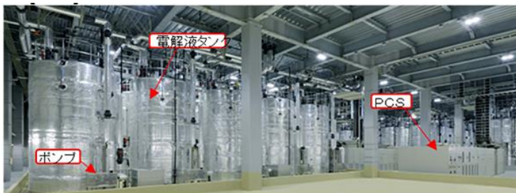
Figure 1: Redox flow battery at the Minamihayarai substation of Hokkaido Electric Power Co.
