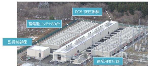
Figure 2: Lithium batteries at Tohoku Electric Power Company's Nishi-Sendai substation
