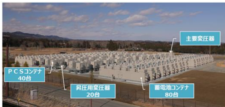
Figure 3: Lithium batteries at Tohoku Electric Power Company's Minamisoma substation
